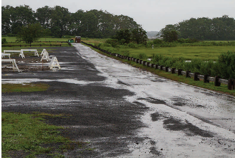
Widening of this drive at the east end of the Meig's Point Nature Center parking lot at Hammonasset Beach State Park elicited a large and concerned response from the Connecticut birding community. Photo by Jack Faller
